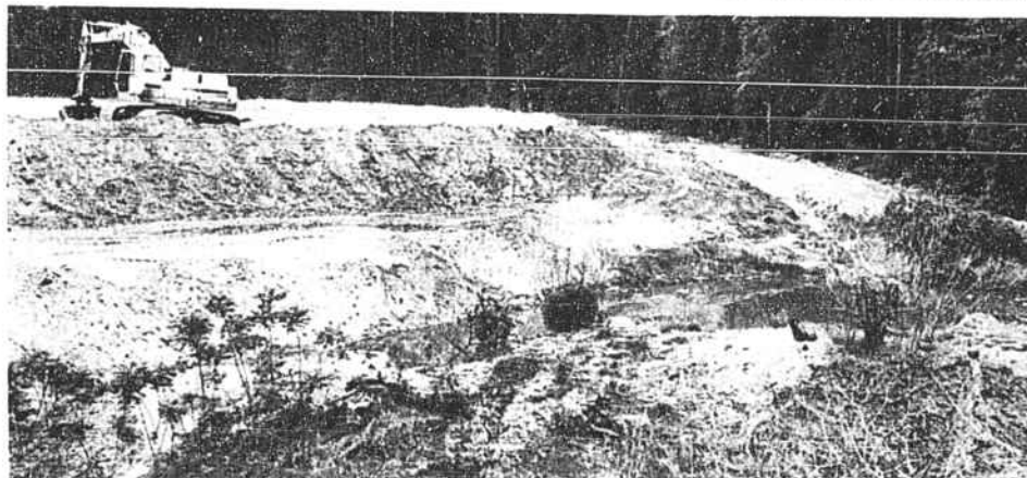
BRUNSWICK COUNTY WAS NOTIFIED last week that it must correct a waste management violation at the Brunswick County Landfill near Supply within 30 days. In March, a waste management specialist from
