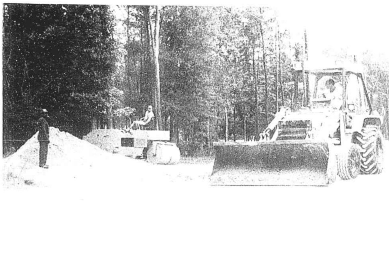
PAUL SCHAFFER of S&W Investments Ltd. uses a backhoe to level gravel on Country Club Drive in Brierwood Estates in preparation for a paving project
