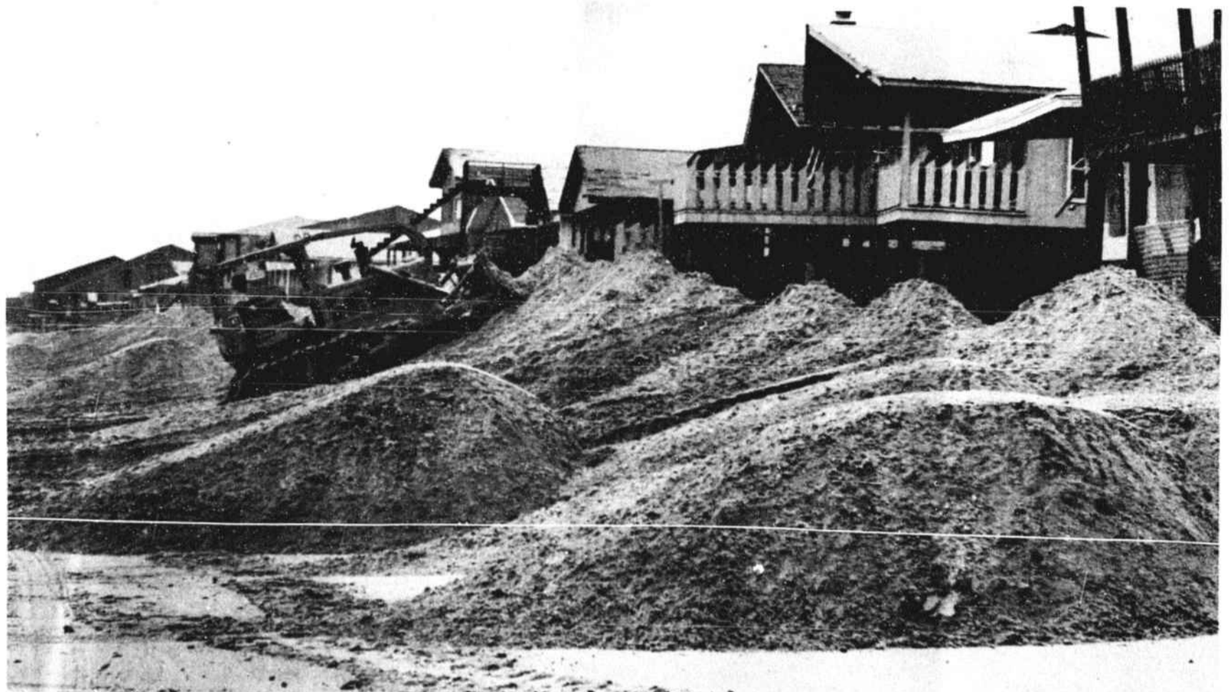
A BULLDOZER CREATES a dune out of piles of sand at the east end of Ocean Isle Beach Saturday in the area where federal officials authorized construction of an emergency berm. STAFF PHOTO BY DOUG RUTTER
