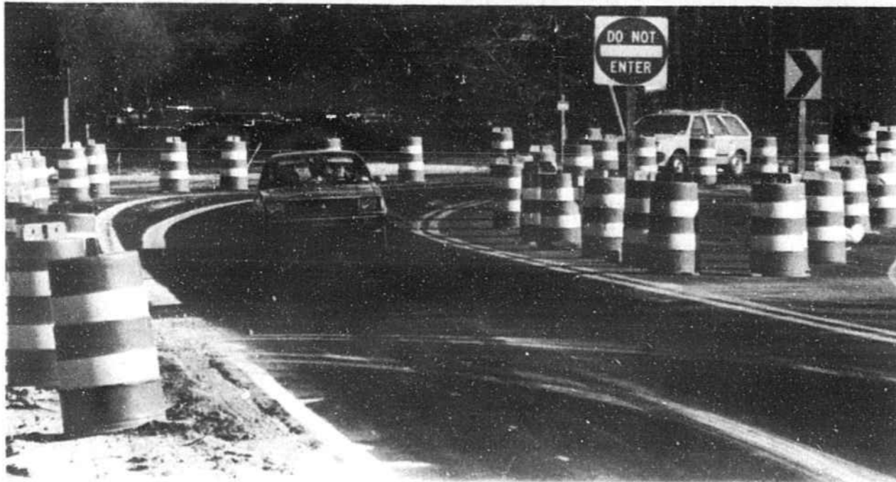
TRAFFIC FLOWED smoothly Monday along the U.S. 17 detour route on Red Bug Road north of Shallotte. An accident on the route Friday resulted in hit and run charges against one driver. The Shallotte bypass is scheduled to open by Memorial Day weekend.
