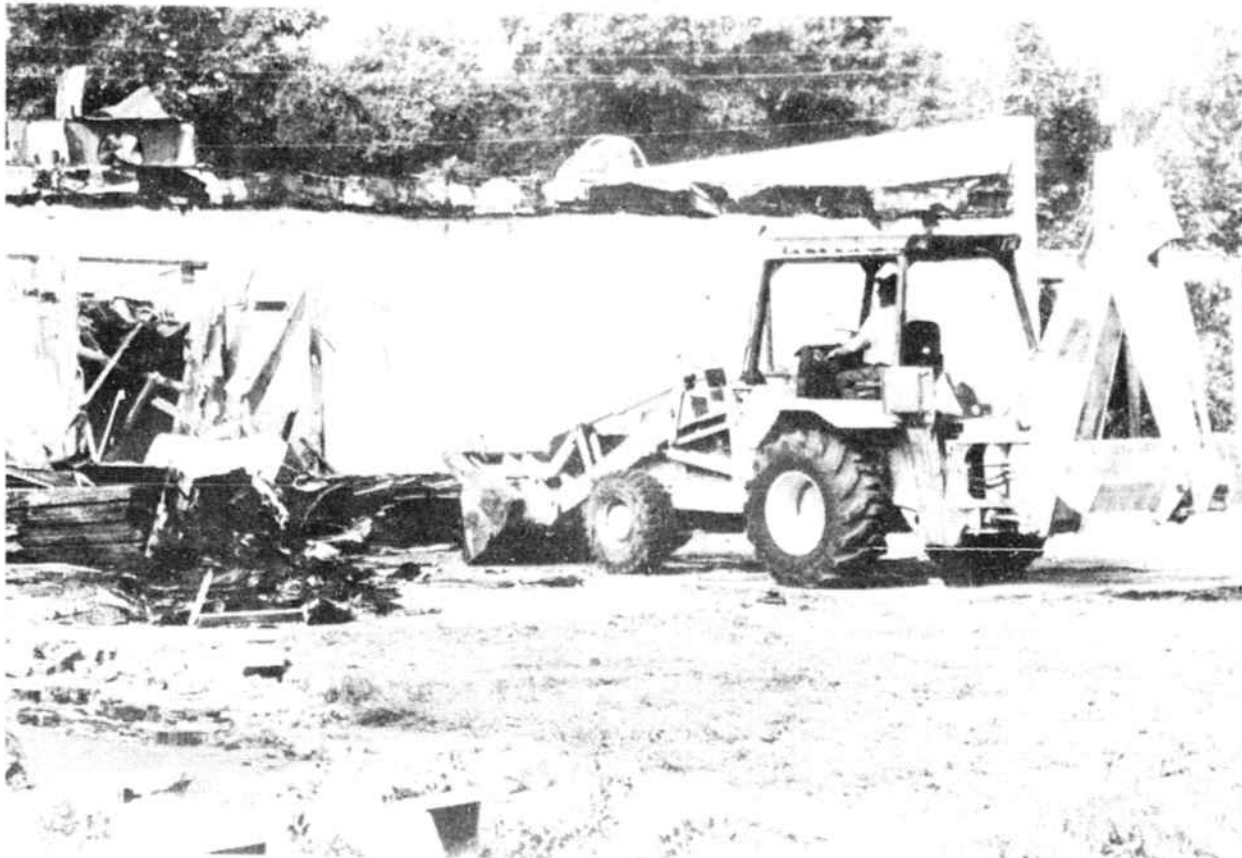
BRUNSWICK COUNTY Building and Grounds employee Wayne Lewis uses a backhoe to demolish the old Bolivia Plaza.
