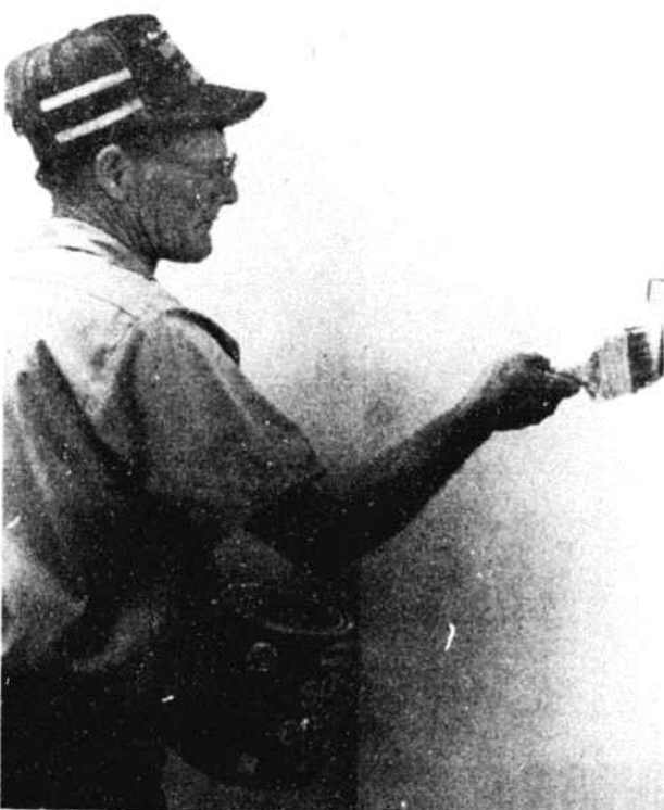
PAINTER BOBBY MILLS adds a fresh coat to the old Department of Social Services building.
