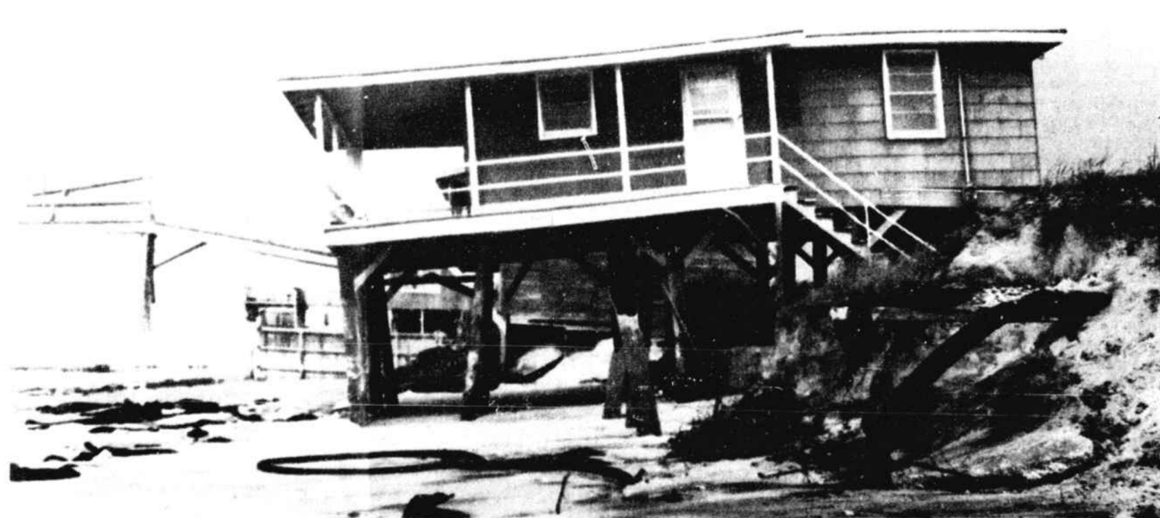
THE MITCHELL HOUSE at 232 Hillside Drive, Holden Beach, was leaning toward the ocean before Hurricane Bob passed offshore Sunday. The storm caused some minor erosion near the east end of the island where this cottage is located.
