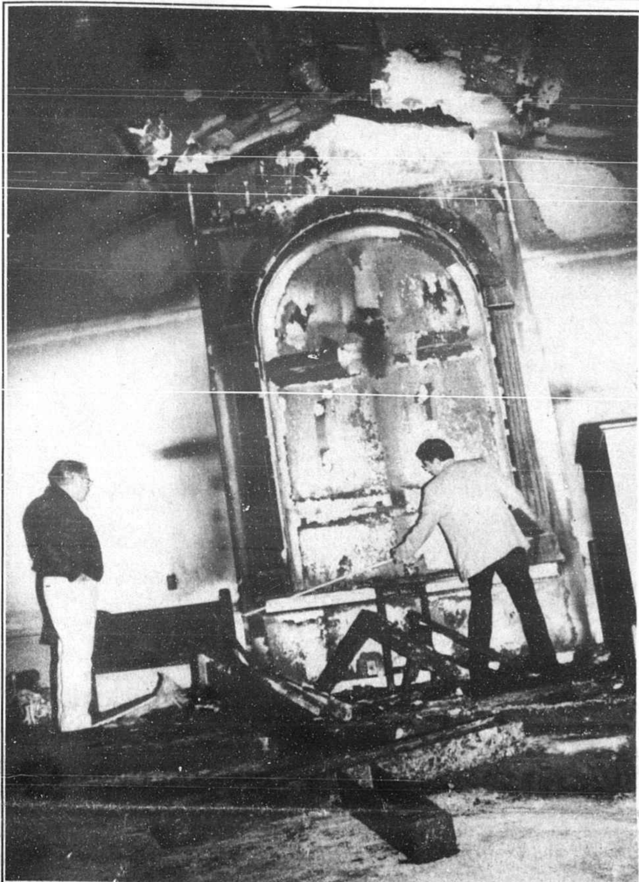
SESSIONS MEMBER JIM INNES (left) looks on as insurance adjuster Dave Morris takes measurements and compiles information in the aftermath of a fire Saturday that damaged the fellowship hall and temporary sanctuary of Shallotte Presbyterian Church.
