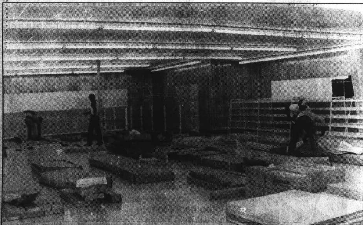
Workers were busy last week at the new Family Dollar Store in Alliance setting up the shelving and other fixtures. The store is scheduled to open Thursday, November 20, with a ribbon cutting ceremony at 10 am. John Marks, district manager, was at the store last Thursday interviewing prospective employees; twenty-one were hired for the temporary stocking and setting-up positions. The manager will be Janice Popper who is being transferred to Alliance from another store.
