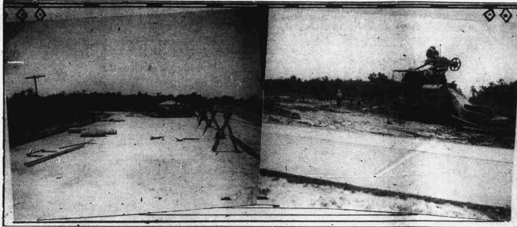
Section of newly-built roadway showing approach of highway to Albemarle Sound bridge for U. S. 17. Left is from north and right is junction from the south when it was being completed.
