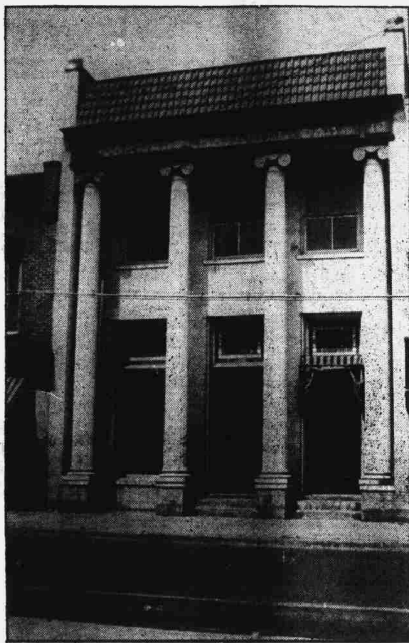
The new United States Post Office quarters in Hertford on Church Street. Alterations are underway and the new quarters will be ready for occupancy in September.
