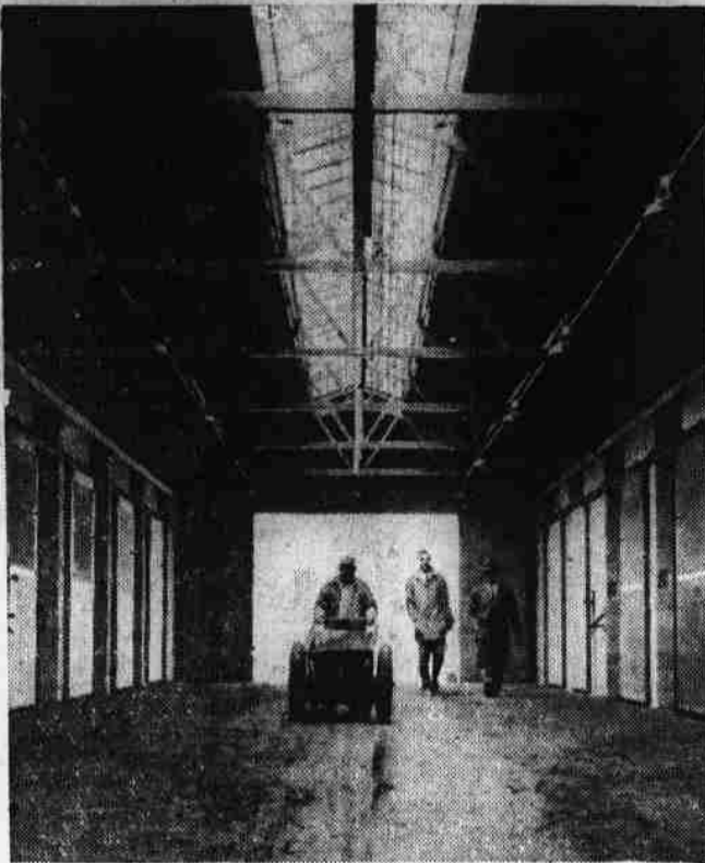
DE LUXE HORSE HOTEL — Carpeted with 10 inches of packed dirt over four inches of gravel, portion of horse barn pictured, above, is only a small part of a de luxe horse hotel for the elite of the equine world now under construction at Yonkers Raceway, Yonkers, N.Y. Eight 84-stall, two-story barns will be in the group. "Apartments" on second floors will be staggered so that guests walking above won't disturb the temperamental occupants of first-floor "suites." Plans will lead to the second-story accommodations. Cost of the project: About $2,700,000.
