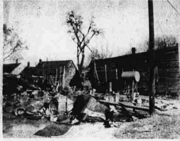
The big cleanup is going on at the end of Church Street in Hertford with the demolishing and cleaning up of the old frame houses that have stood at the South end of town for many, many years. They were occupied for years by many Negroes that were employed at Major Loomis Lumber Company and Southern Cotton Oil Co. when the two businesses were here.
