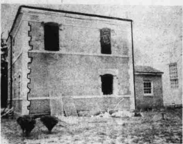
WORK CONTINUES - Progress on the demolition of the Perquimans County Jail continues. This past week, the windows were torn out, leaving the appearance of a bomb going off in the structure. The jail was built between 1900 and 1906. (Staff Photo By Francine Sawyer)
