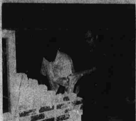
PILING IT ON —The two men in the foreground skillfully add another layer of brick while instructor Askew looks on. Brick masonry is one of the many adult education classes being taught at Perquimans County High School.
