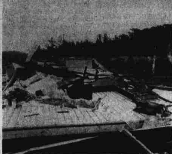
destruction. Bremus, a native of Virginia, had the trailer moved to Holiday Island two weeks before the disaster. He
