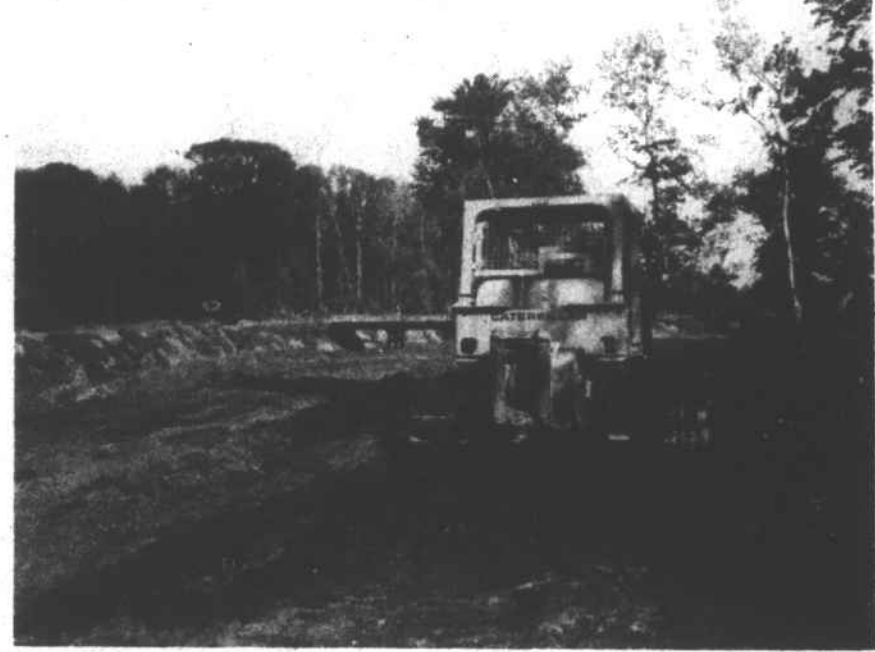
OFF MONTH WORK — Travelways on much of the Bear Swamp main channel have been smoothed and seeded during April and May since biologists agreed that excavation during those months would have been detrimental to wildlife there.
