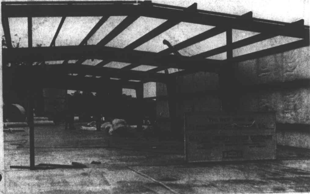
REBUILDING UNDERWAY — Farmers Feed & Seed Company will soon be returning to its Grubb Street location with the completion of a rebuilding phase. The local business was destroyed in the Jan. 10 fire originating at Winslow Oil Company and has since been operating temporarily in Winfall. (Staff photo by Paige Eure)
