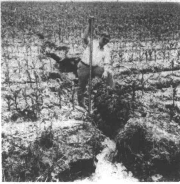
WASHOUT — David Leatherwood inspects cross drain that has washed out during recent heavy rains. (SCS photo)
