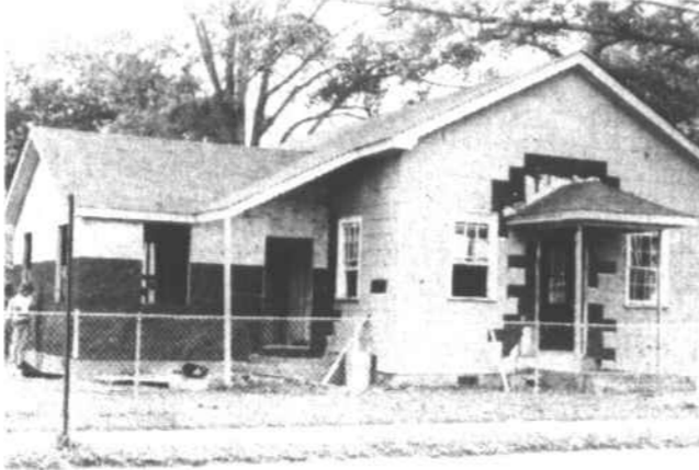
CENTER PROGRESS - Work on the new Senior Citizens' Center is proceeding rapidly. The Center should be ready for dedication in late August or early September. (Staff photo by JACK GROVE)
