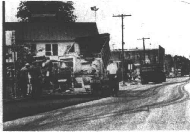
PAVING GOES DOWN — This was the scene on Church St. Wednesday, June 27 as state highway crews paved the street surface from U.S. 17 Bypass to Dobbs St. (Staff Photo by JACK GROVE)
