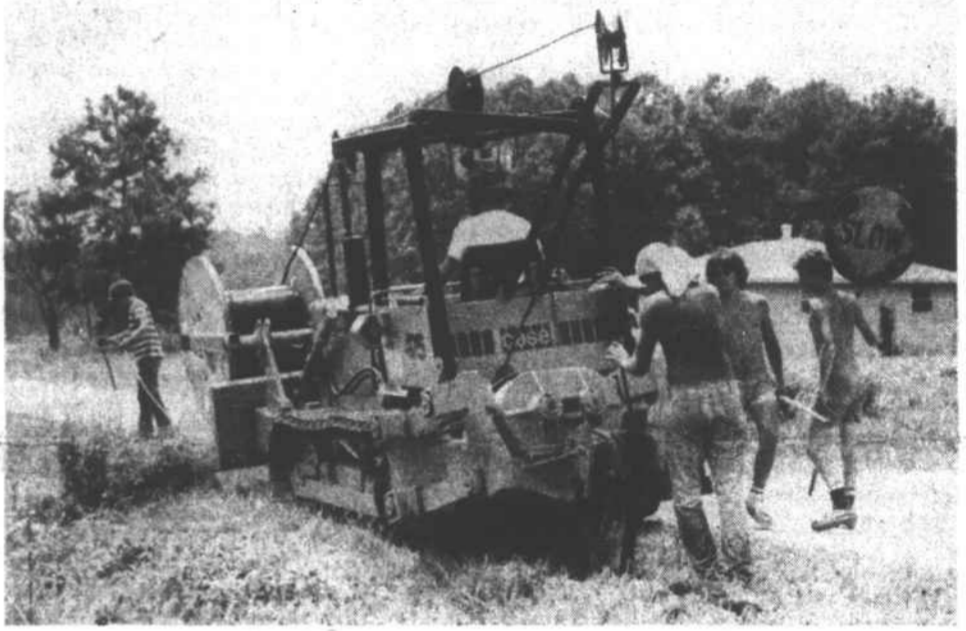
NEW PHONE CABLE — A crew lays a "relief cable" in an operation that has been worked on for about six weeks. The cable is being laid from Highway 17 out the Harvey's Point Rd., across to the Holiday Island Rd. and into Holiday Island. The specially designed tractor digs a two foot deep trench and lays the cable in one continuous operation. The new cable will make possible the installation of between 100 and 200 new phones at Holiday Island.
