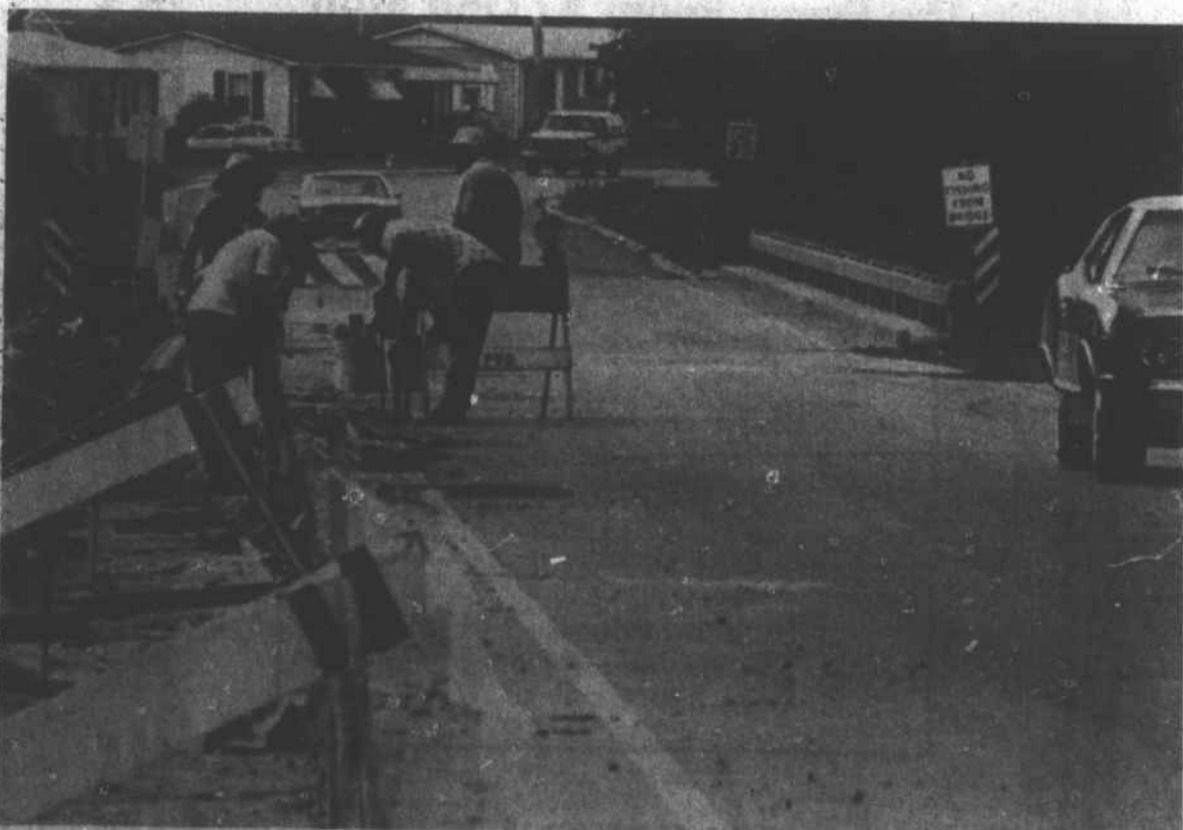
Road workers defy the heat while constructing curbs along Church Street in Hertford. The National Weather Service expects hot, humid weather to continue through the weekend.
