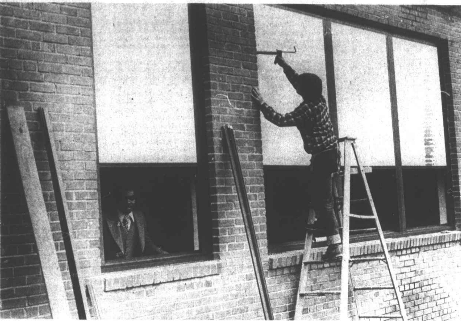
The windows have arrived for the window replacement project at Perquimans Union
