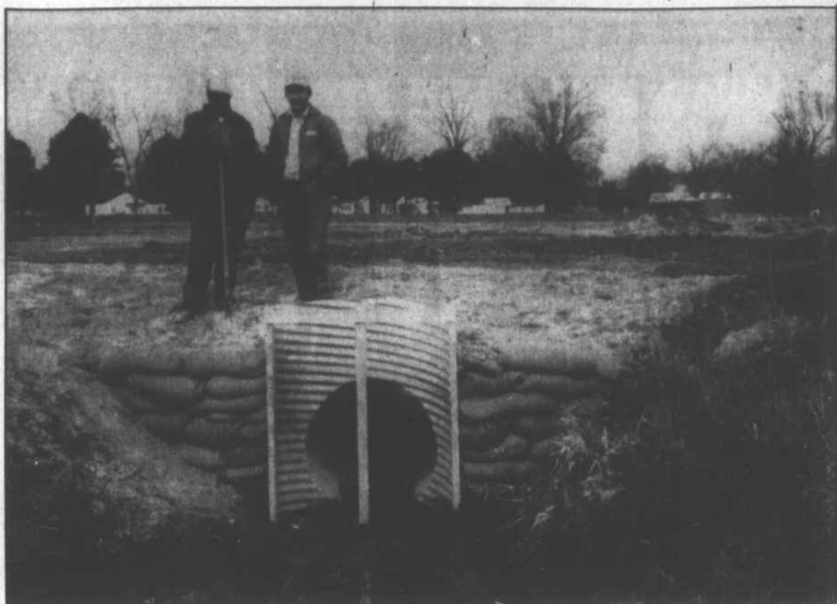
Ed Nixon and Watson Blanchard inspect a recently installed water control structure on Nixon's farm.
