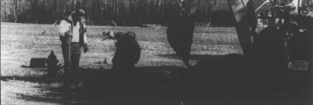
Members of the Perquimans County Water Department maintenance staff work in the New Hope area of Perquimans County installing a water tap.
