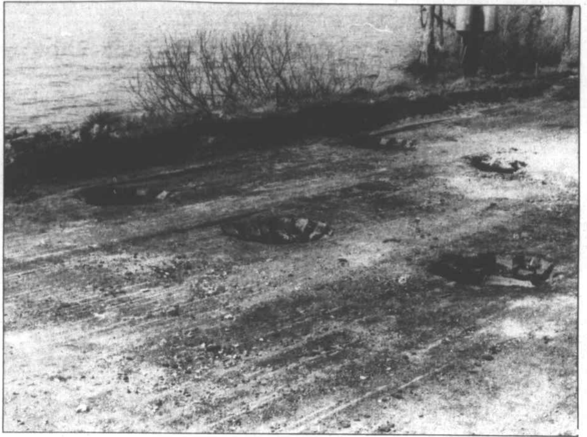
Highway workers on the causeway project have drilled huge holes in the old road bed. Steel pilings are being driven through them to anchor the new road.
