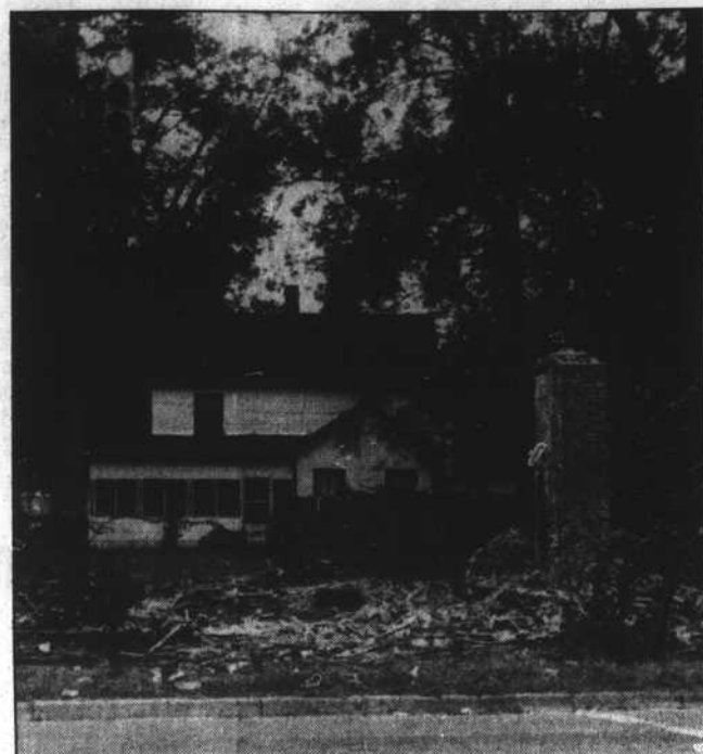
The house that once sat on the corner of Edenton Road and Market streets has been dismantled. All that is left of the former dwelling is part of the chimney and debris. The property, which is owned by the Bertha C. Lane estate, was one that the town had targeted for condemnation.
