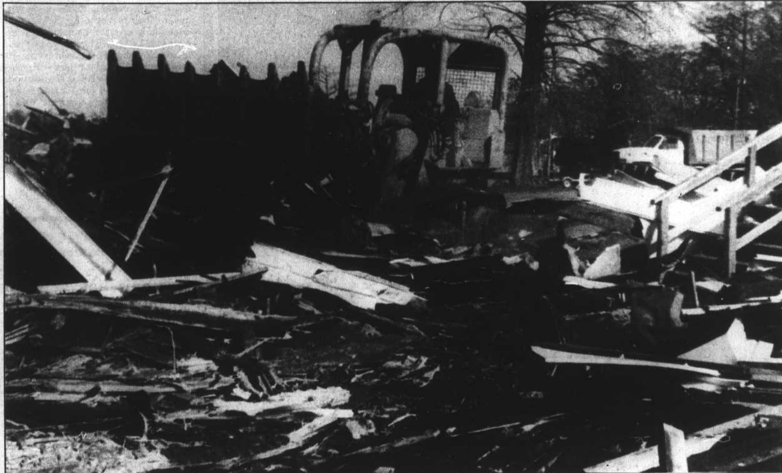
The town of Hertford recently hired clean-up crews to demolish what was left of the former police station. The plans being drawn call for the building to be reconstructed on the same site and to be larger than the former building. The town council should review the tentative plans by next week.
