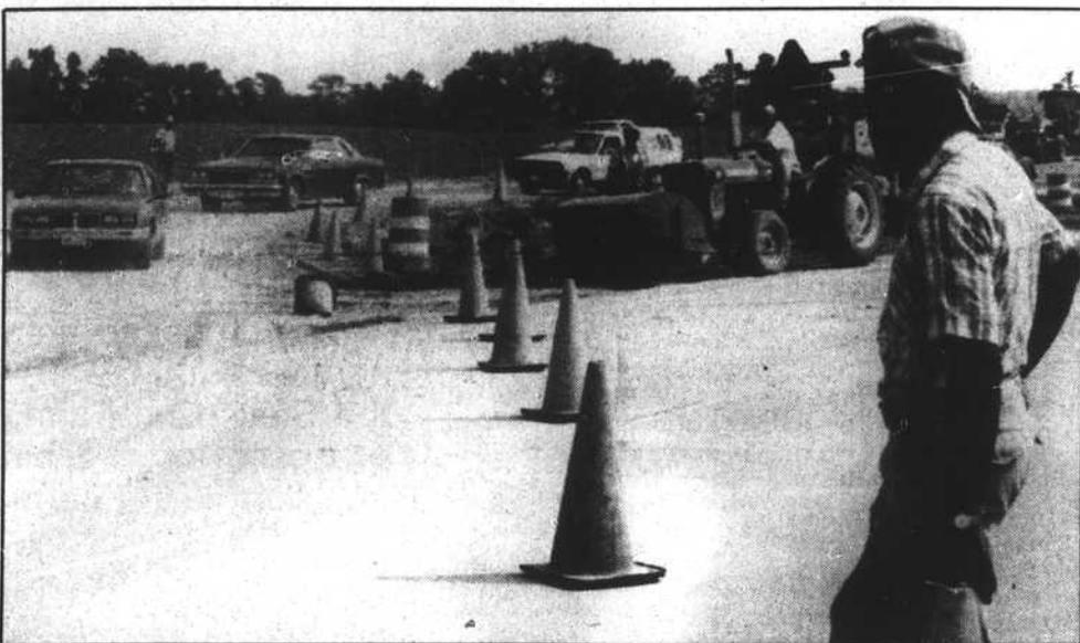
Traffic detours and slight delays are the price of progress along U.S. Highway 17 Bypass from Winfall to just south of Hertford. DOT officials said last week the four-laning project is ahead of schedule. The new bridge, however, will not open until late 1994.
