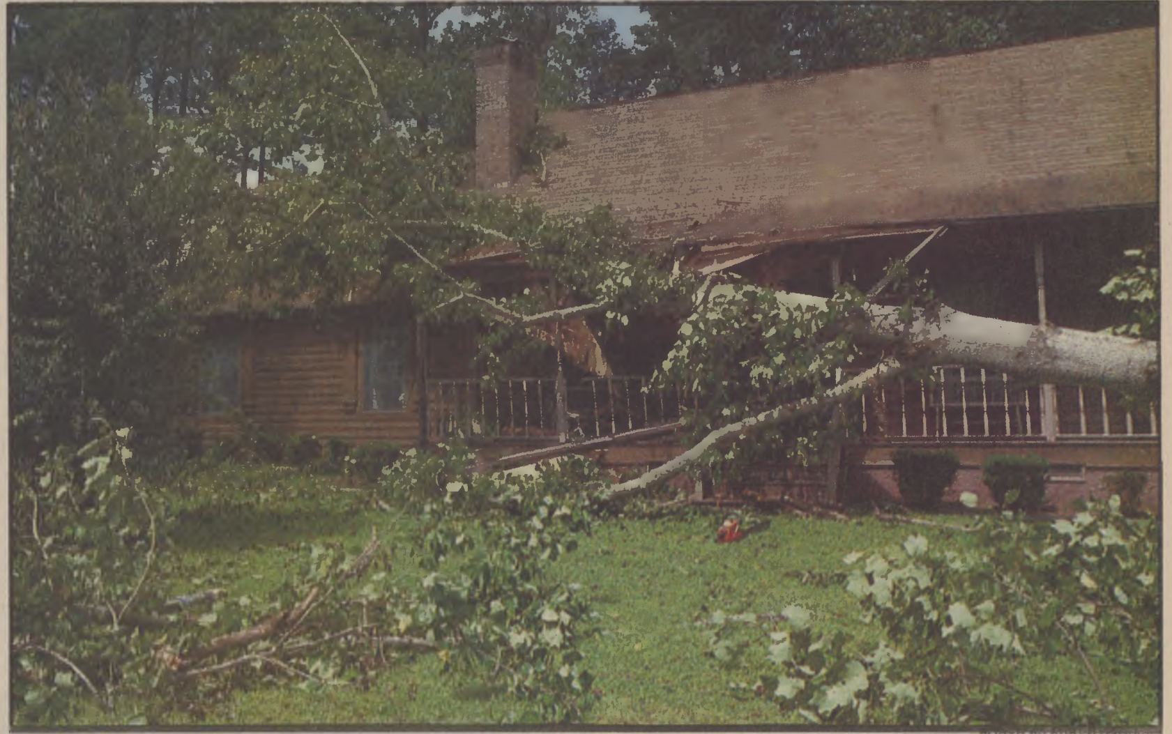
The Sunset Drive home of Lizzie Harrell sustained damage Thursday night when Hurricane Fran blew through North
