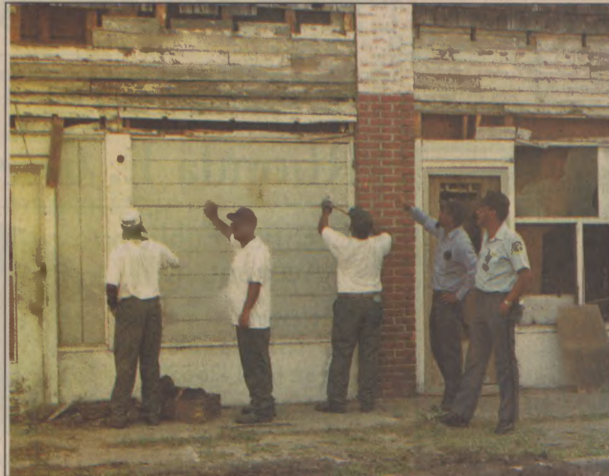
Inmates from the Gates County Correctional Facility begin cleaning out the Keel building on the corner of Edenton Road and Grubb streets. The work crews emptied the building's contents last week and cleared the area around the building in preparation for demolition.
