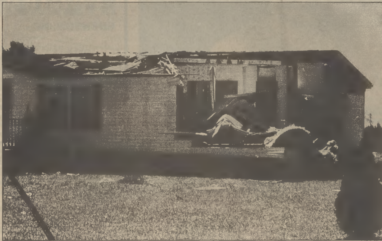
A tornado touched down in the Durants Neck area of Perquimans County late last Wednesday night, damaging three houses. Among those damaged properties was the doublewide mobile home of Jeff and RoseAnn White. The right front wall was ripped from the home, exposing clothes hanging in the closet.
