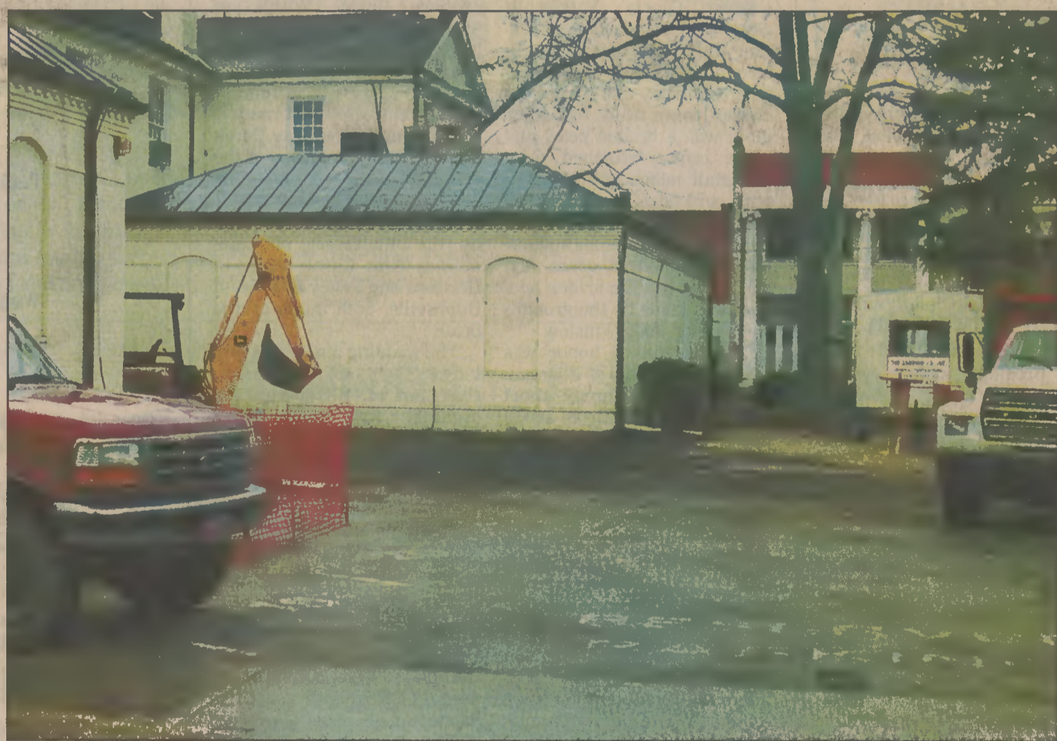
Work has begun on the additions to the Perquimans County courthouse. Wings will be added to both sides of the structure, adding much-needed space to the Clerk of Court offices as well as an elevator to the second floor and public restrooms that can be used for festivals and other community events downtown.
