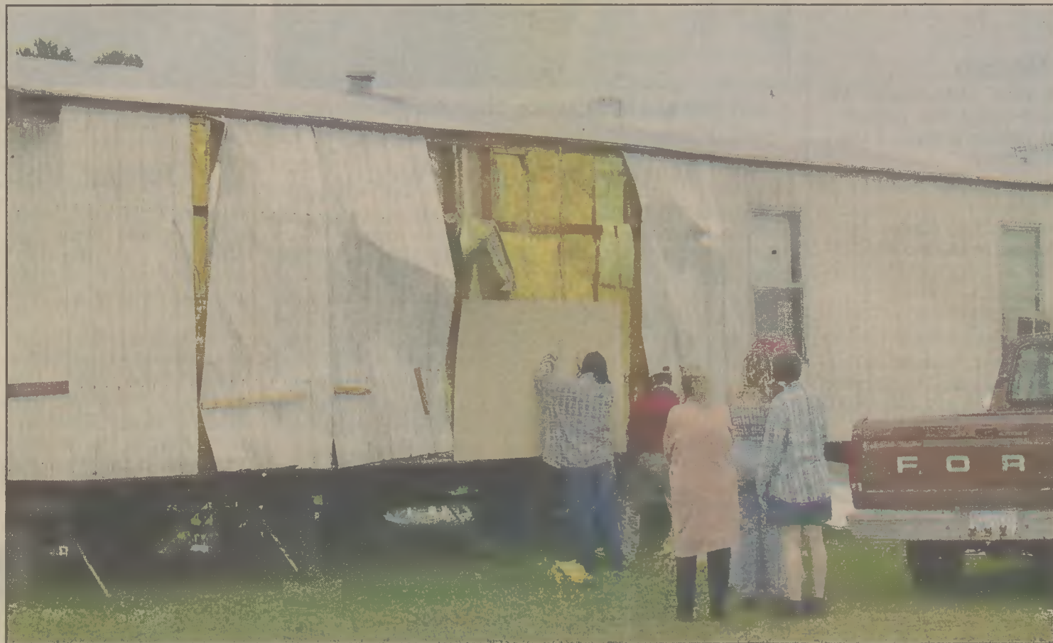
Family and friends try to cover the damage done to the mobile home of Richard Gilbert after Friday's thunderstorms, which spawned strong winds, ripped through Miller and Meads Mobile Home Park. The winds cut a swatch about a mile wide, starting behind the Riverwind Subdivision and stretching north to Belvidere Road and south to Ballahack Road. The wind moved all the way through Hertford and Winfall.
