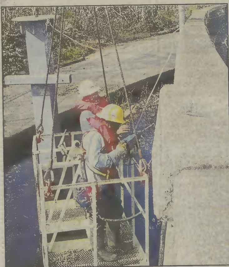
Employees of Lee Construction Company are lowered in a steel safety cage over the side of the S-bridge, where they complete part of the work necessary to install the period lighting on the historic landmark. The bridge will be closed at least until Friday as the work continues.
