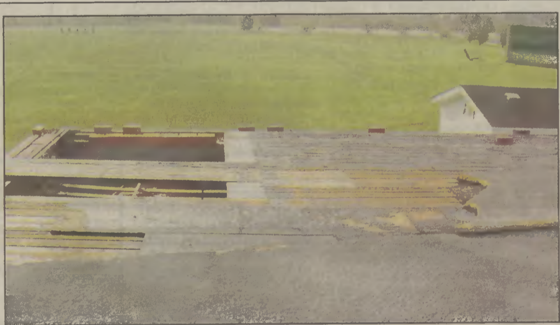
The roofs on the buildings at Perquimans County Middle and Hertford Grammar schools need replacement, school officials say. The roofs were already in need of renovation when Hurricane Isabel came through in September and did extensive damage at Perquimans County Middle School.
