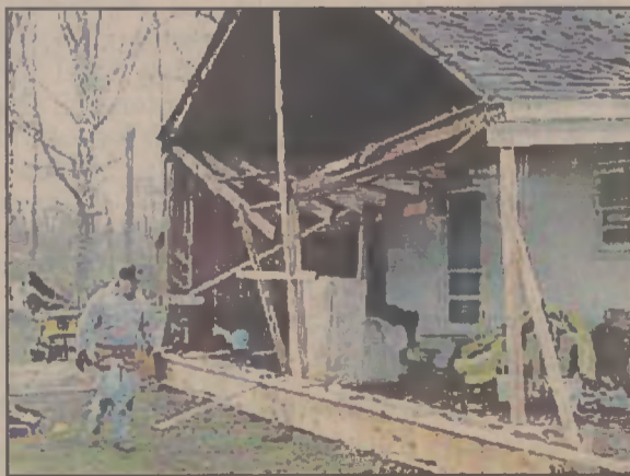
Hurricane Isabel blew through the Albemarle area with a fury, damaging thousands of homes throughout the area. The M.E.R.C.I. Northeastn Diaster Recovery Center in Edenton is helping those unable to afford home repair.
