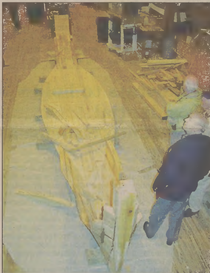
The historic construction of the periauger, a Colonial era log boat, is being beamed worldwide by a webcam installed at the N.C. Maritime Museum's Watercraft Center, the site where the boat is being built. The progress of the boat's construction can be viewed at the site www.estuarylive.org .
