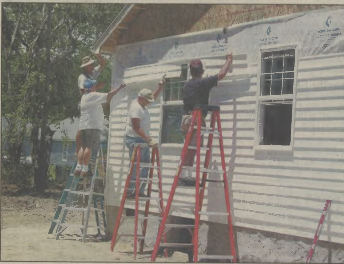
Work is in full swing at the Habitat for Humanity house being built in Snug Harbor. On Monday, volunteers were installing siding while heavy equipment operators were in the back yard putting in the septic system.
