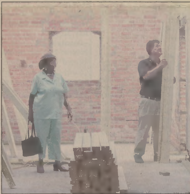
Randy Lassiter, owner of the building at the corner of Grubb and Edenton Road streets commonly known as the Keel Building, shows Hertford resident M.B. Taylor how work is progressing at the site.
