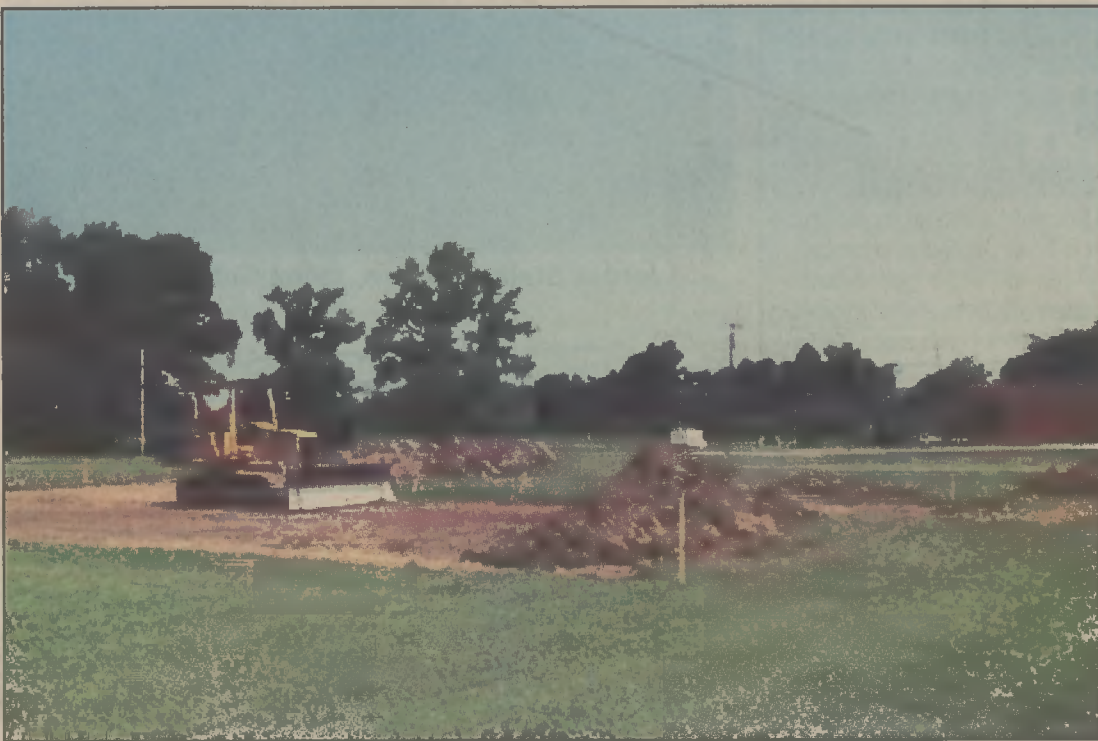
Construction has begun on moving Jimmy Hunter Drive south to make way for the new high school gymnasium.
