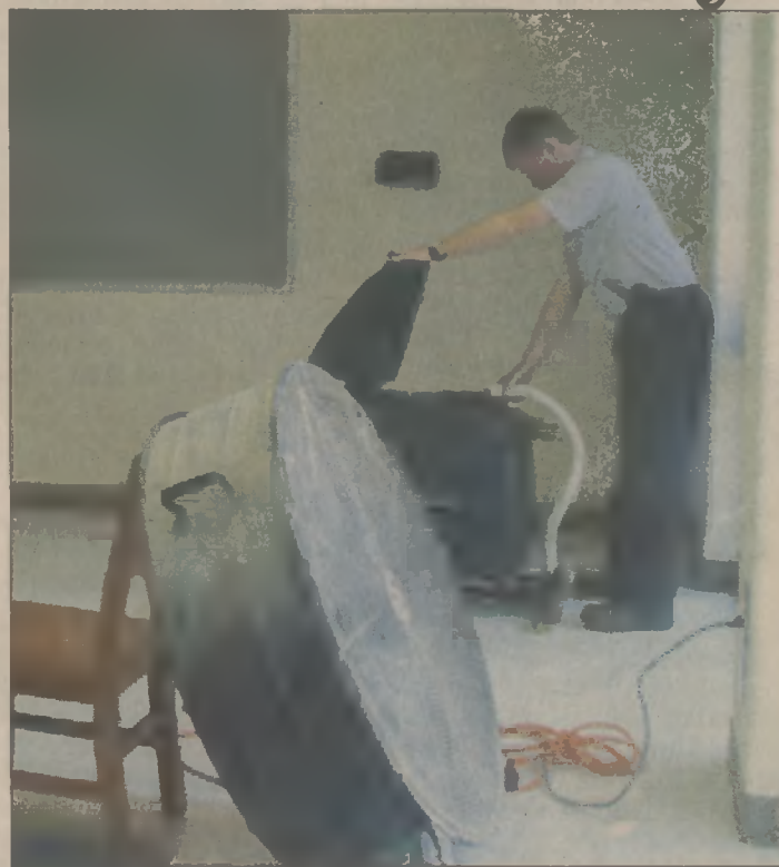
Perquimans Weekly photo by CATHY WILSON JONATHAN NIXON, DIRECTOR OF maintenance, checks the machine that eliminates any water on the classroom wall following last week's fire on the roof connecting the new gym to the old school.
