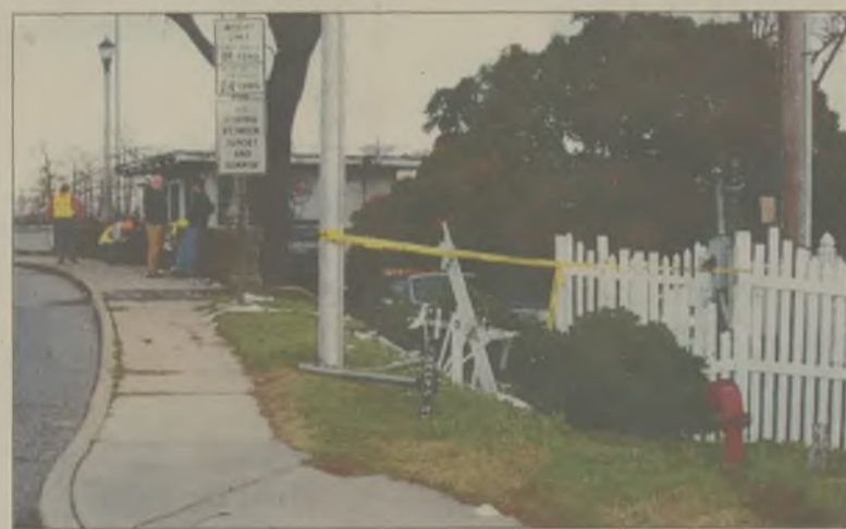
N.C. Department of Transportation workers inspect the S-bridge after a pickup truck ran off Church Street, crashed through a fence, struck the bridge and hit the bridge tender's house, before plunging into the Perquimans River early Saturday.
