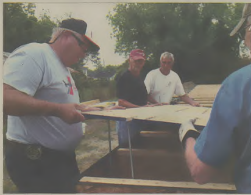
Volunteers Frank Elfring, Don Locascio and Skip Matthews lay flooring on a new Habitat for Humanity house on Dobbs Street in Hertford last month.
