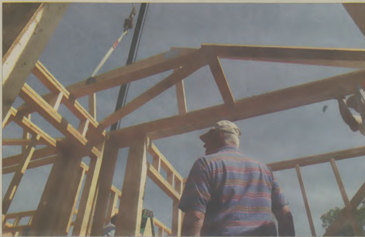
A Habitat for Humanity volunteer watches as a crane positions a roof truss onto a home under construction at 317 Dobbs St. in Hertford last week.
