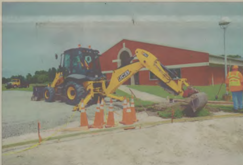
An N.C. DOT backhoe moves sod to make way for a concrete sidewalk at Perquimans Central School last week.
