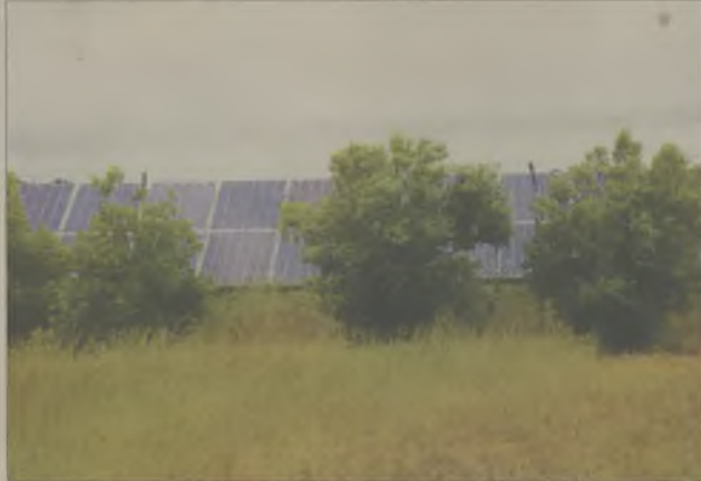
STAFF PHOTO BY PETER WILLIAMS Plants partially buffer a solar power project on Belvidere Road. The Perquimans County Commission has enacted a second moratorium so the rules can be amended to make sure developers in the future provide buffering.
