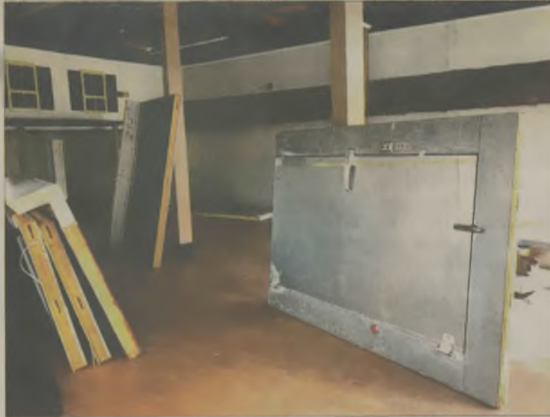
A walk-in cooler waits to be assembled at the Hertford Bay Taphouse.
