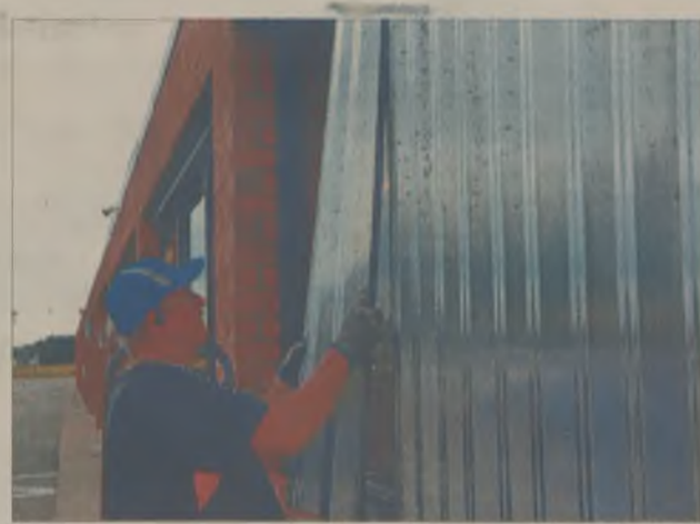
Johnny Greene puts up metal storm shutters Thursday morning at the Food Lion store in Hertford. The store was open, but had few shoppers at the time.
