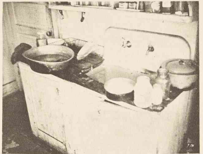
Stopped-up Kitchen Sink
