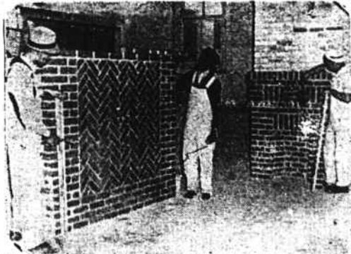
A. and T. College, Greensboro, N. C., is doing her share in preparing skilled workers for the national defense program. A herringbone panel and a chimney, fireplace and brick mantel are being completed by these students of a brick masonry class. They are, from left to right: Alus Richardson, senior brickmason, from Apex, N. C.; Edgar Murphy, Kingston, N. C.; and William Lee, Springfield, Ill. All three are honor students.
